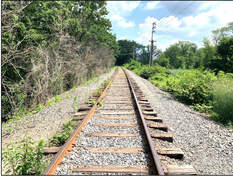
Typical tie, rail, ballast, and vegetation conditions on the Southern Branch between Farmingdale and Lakewood, NJ.
