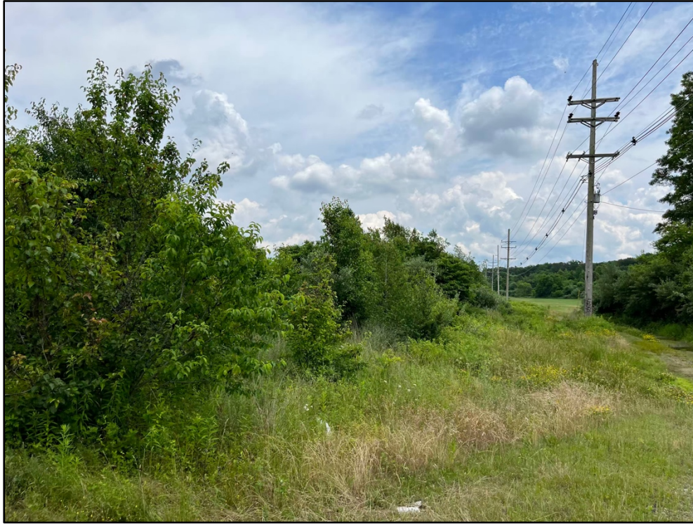
View of F&S Connection right-of-way at Oakerson Road facing east toward Farmingdale showing typical heavy vegetation growth. Track is removed a distance of approximately 100' from public roads, but is otherwise in place.
