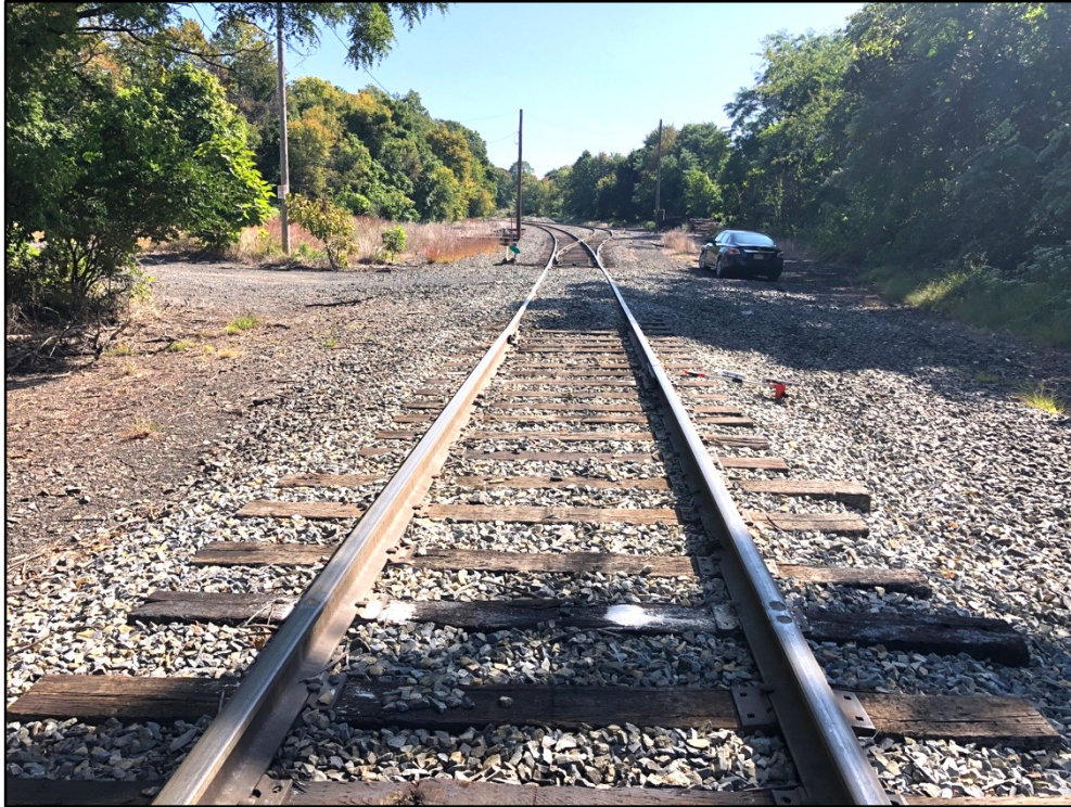
View of Dover & Delaware Eastbound main track, facing east at Stockton Street, at the location of new left hand turnout and corresponding left hand split rail derail.
