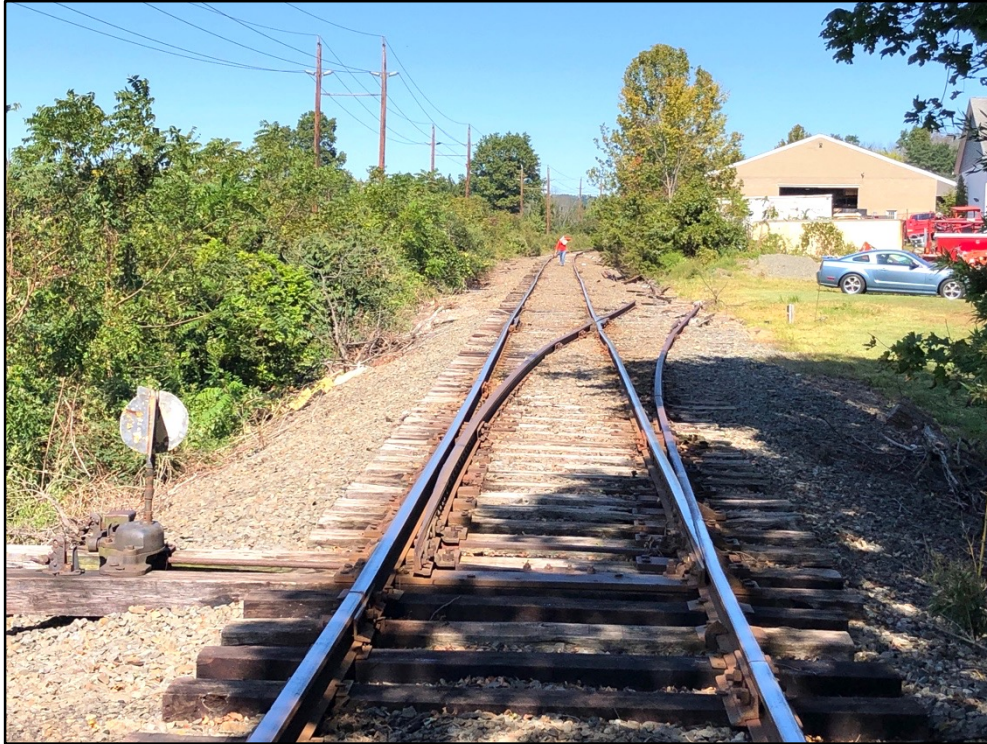
View of Black River & Western Railroad No. 8 turnout at south end of Copper Hill siding to be replaced with a No. 10 turnout at the same location.
