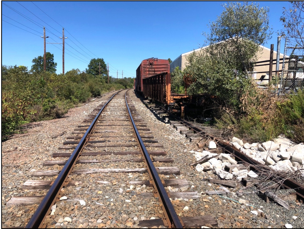
View of Black River & Western main track facing north with the existing siding on the east (right) side. Existing siding shall be removed and replaced with 100#PS rail and wood ties salvaged from Schedule F work.
