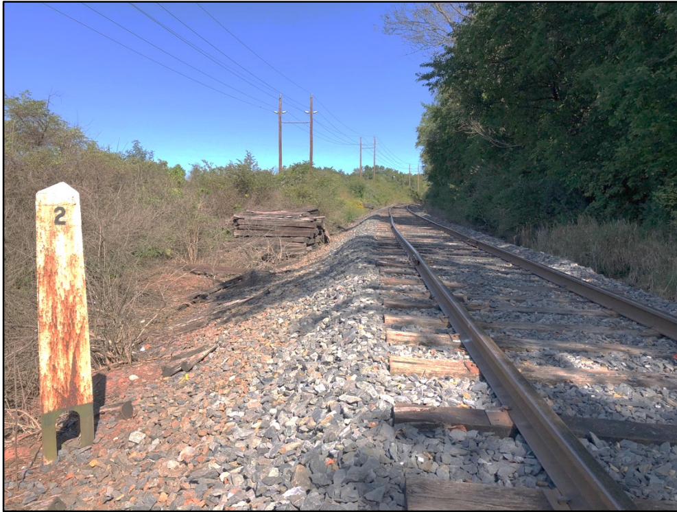
View of Black River & Western main track facing north at Milepost 10. Existing track shall be removed and replaced with 132#RE rail on steel ties., west.
